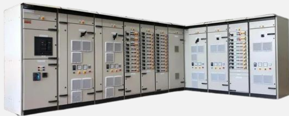
Switchgear and skids
