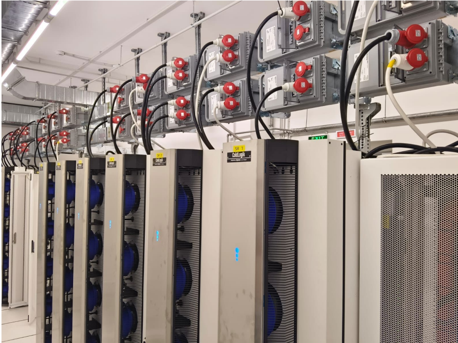
ColdLogik Active Rear Door Cooler (RDHX) from USystems (a brand of Legrand) at Yerevan State University (Armenia)
